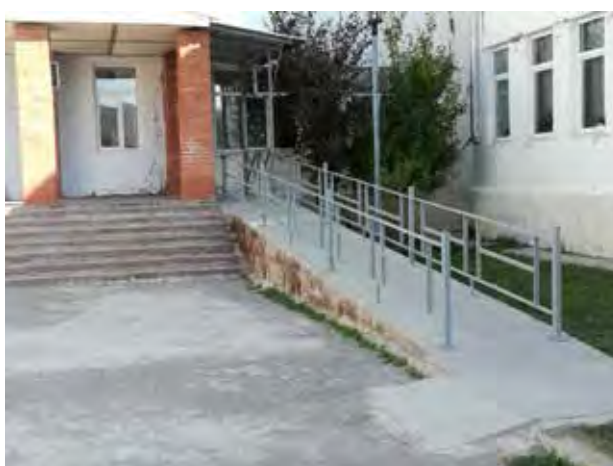
Picture 1 © Flieger: All participating schools were supported to make schools more accessible for persons with disabilities, e.g. by building or renovating ramps.
